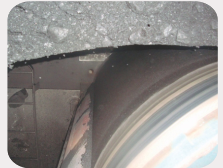
Super-Skalper IV 72" system installed on this coal handling conveyor belt at this major coal-fired plant.
