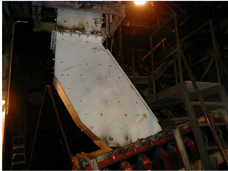
New stainless steel, ceramic lined, “Spooned” for soft loading of the coal in the same direction of belt travel.
