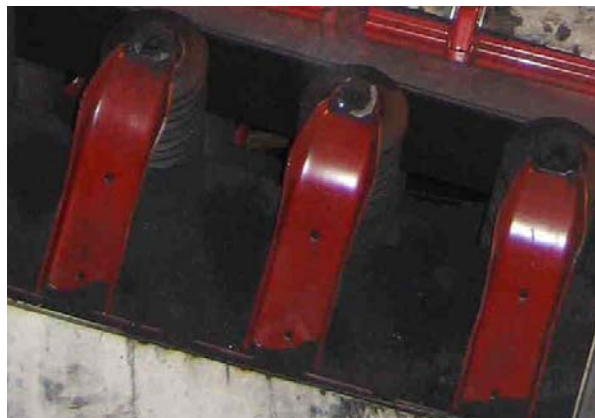
Coal fines and dust building up in between the idlers
