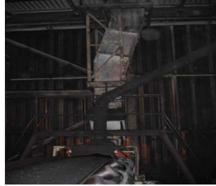
Notice the high volume of dust in the air as the material is loaded on the receiving belt.
