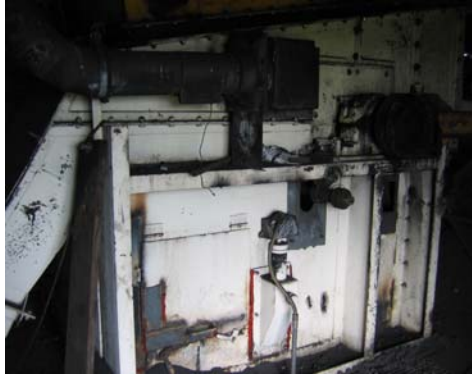
Old and inadequate top half the chute and transfer point.
