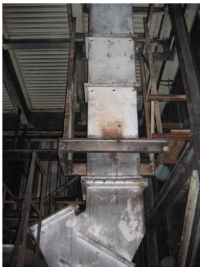
Existing chute with a straight drop from 5A conveyor to 6A
