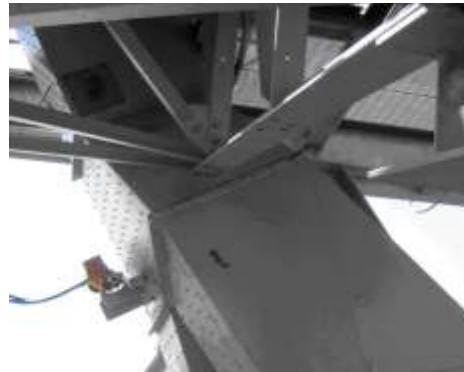
Vibrators and UHMW liners were added with no effect.
