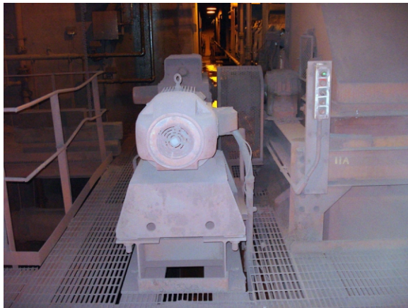
Before - Unguarded machinery
