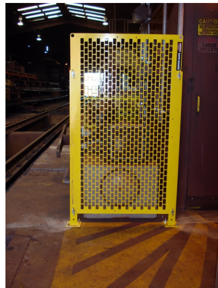
Results - ASGCO® Safe-Guard™ Flat Conveyor Guard protecting workers from moving machinery
