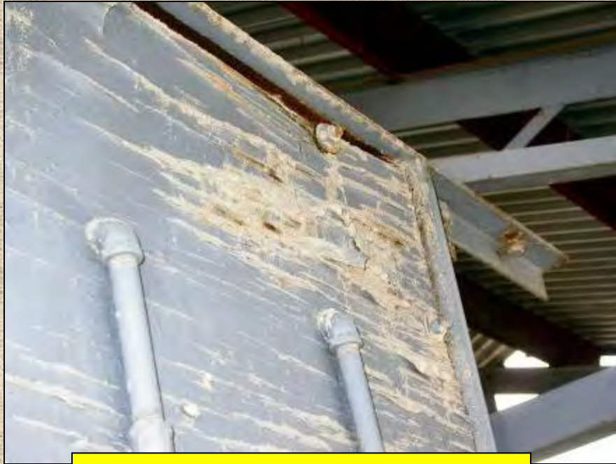
Deteriorating and delaminating
