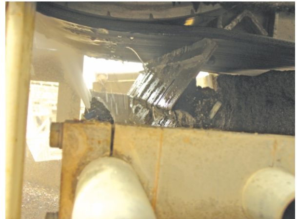
ASGCO Razor-Back with Spray Bar cleans wet sandy carry back from underneath the belt.
