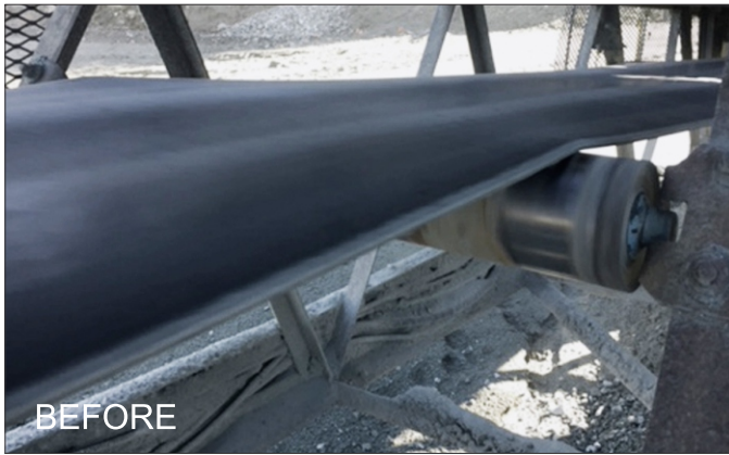
Conventional training idlers installed on non-carrying side pushing belt up with material build-up around the pivot.
