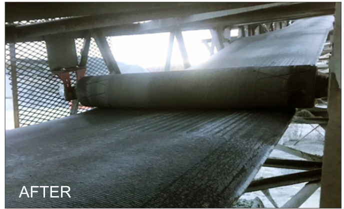
Tru-Trainer® Flat Return Idlers installed on clean side of belt, pushing down to take the tension out and align belt.
