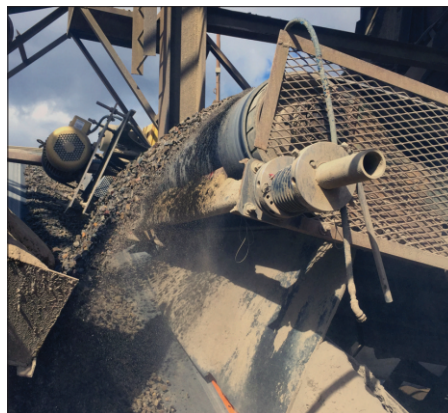
Mini-Skalper ® IV installed on the head pulley.
