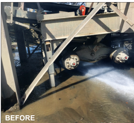
BEFORE Water on the floor from cleaning up the carry-back with high water pressure.
