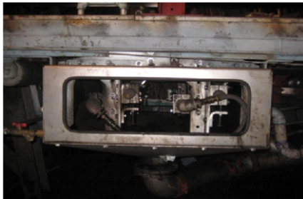
Wash Box Installed
