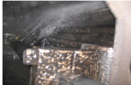
Water Spray Bar Cleaning the Belt
