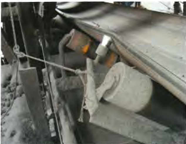
Figure 3. Ordinary training idler tied off with a rope causing material build up on the support frame work and belt edge damage from friction and pressure.
