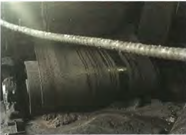
Figure 2. The tail pulley is buried in material.
