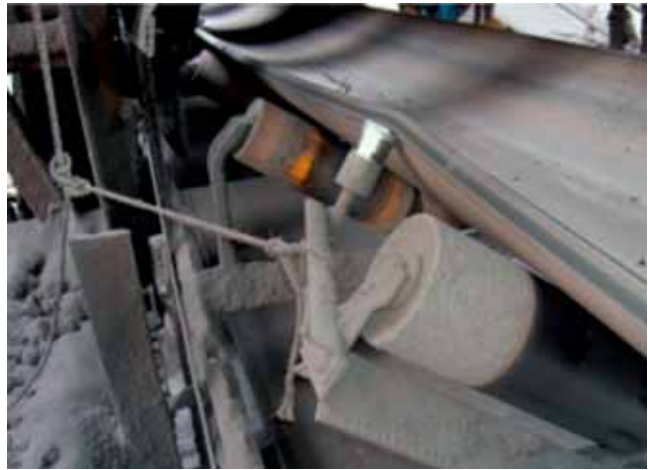
Fig. 3. Ordinary training idler tied off with a rope causing material build up on the support frame work and belt edge damage from friction and pressure.
