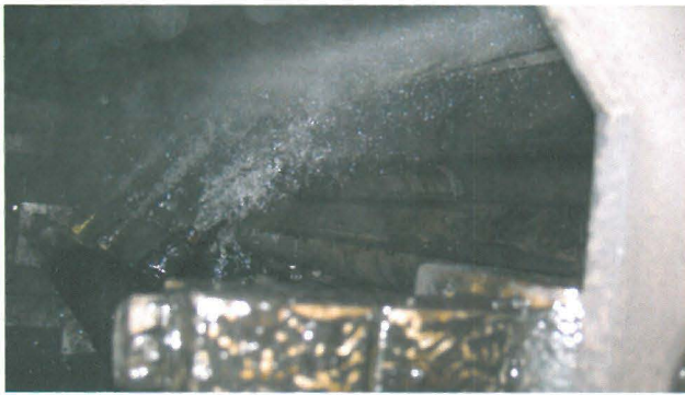
A series of water sprays and tungsten carbide belt cleaners ensure the conveyor belt is cleaned.
