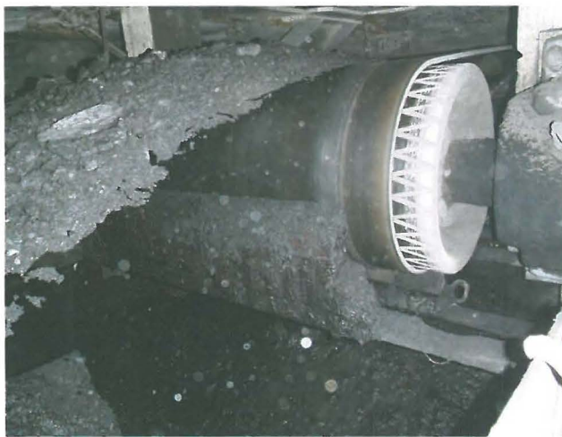
Primary belt cleaner properly installed on this underground head pulley.
