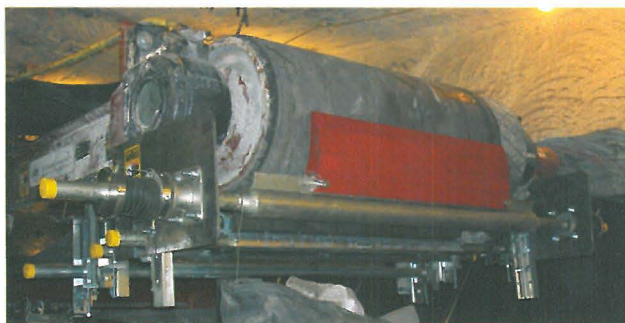
Underground coal mine head section with multiple (4) belt cleaners installed.
