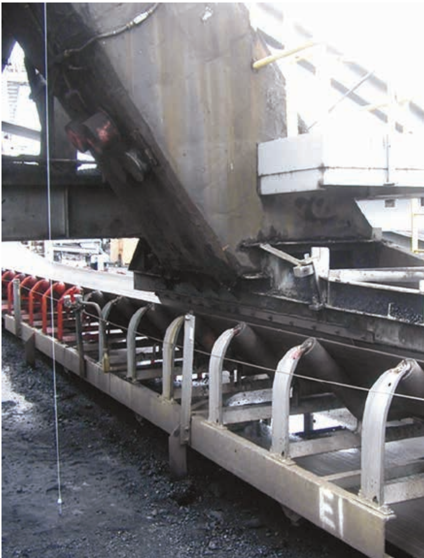
Figure 5. Off-centre loading onto yard belt.
