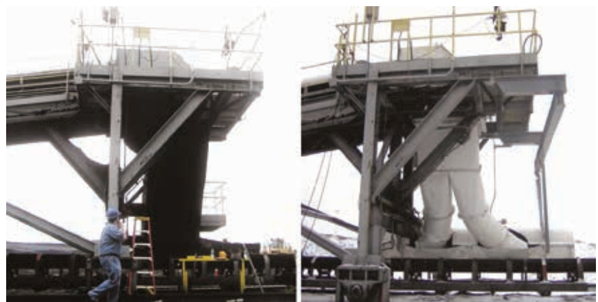
Figure 8. Before (left) and after (right) installation of the new transfer chute with movable deflector gate in the head discharge area and two outlet chutes.
