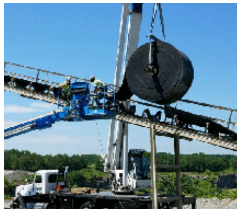
The ASGCO ® service team uses a high reach man lift to lay the belt onto the conveyor.
